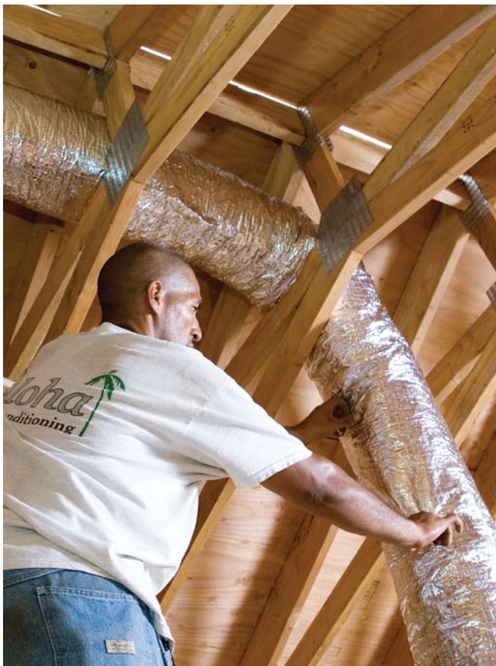
An Aloha Air Conditioning technician runs flex duct to the Fujitsu unit's main multizone air handler.
