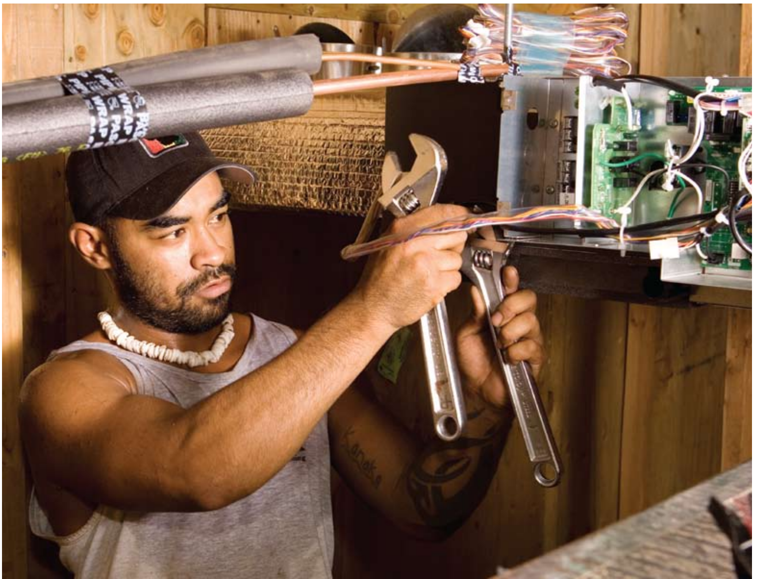
Kaeo Kauai, Aloha A/C installer, attaches refrigerant lines at the air handler hidden above the great room ceiling.
